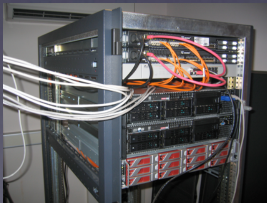
P2SC servers at ROB
